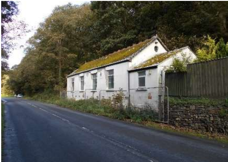
FIGURE 80 THE INSTITUTE IN DISREPAIR
