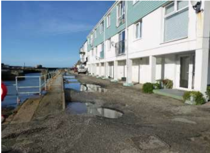
FIGURE 36 POT-HOLED ROAD ACCESS TO NORTH SIDE PARKING AND BOAT STORAGE AREA
